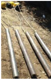
lead wires (Black) and lowering rope (yellow),
