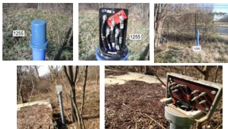
Typical installations of post mount test stations, and test lead wires attached to terminal board. Upper location shows a test station with magnesium anodes installed.
