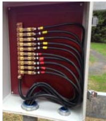
Anode junction box with individual anode leads (red and yellow tape). Single wire on left is anode header cable.
