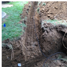
Structure negative lead trench to rectifier
