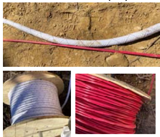
Ribbon Anode and Header Cable (Red)
