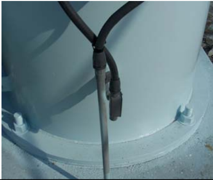
AC and DC wiring
