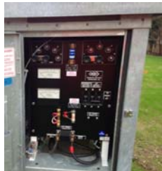
Rectifier close up with anode header cable (red tape) and structure negative lead.
