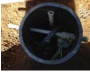
Anode lead wires at top of well and top of vent
