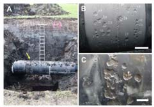
External corrosion on buried gas transmission pipeline in bog soil of Germany.
