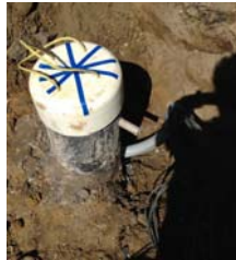
Anode well with vent cap attached, and anode leads in conduit for placement in junction box
