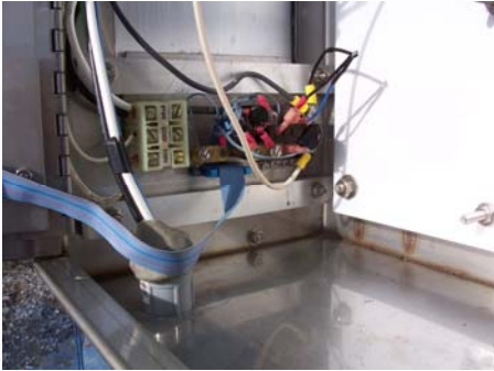
Solid State Rectifier module and feed wires
