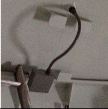
DC Junction Box and PE
