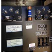
Front panel of rectifier showing Tap settings which control output, volt and ammeter, on and off switch.
