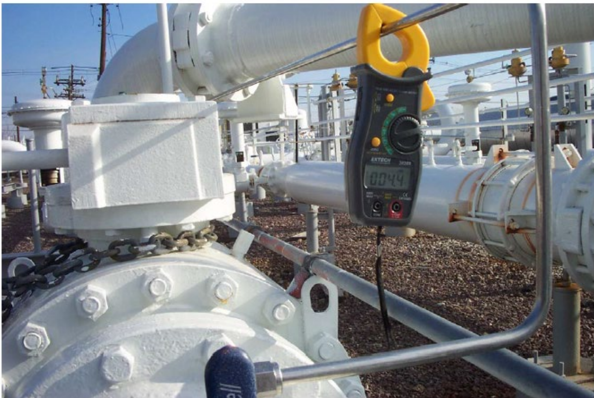
Figure 6-9: Clamp-On Ammeter Measuring Current on Stainless Steel Tubing
