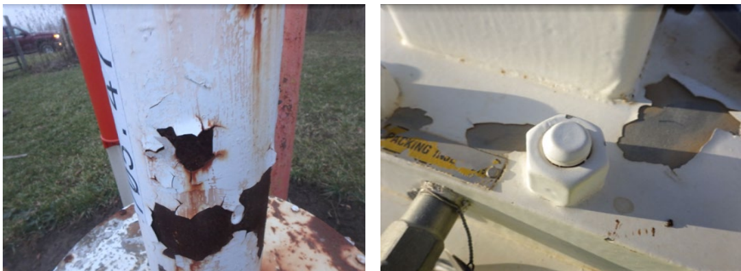
Figure 9-4: Coating Delamination to Substrate
